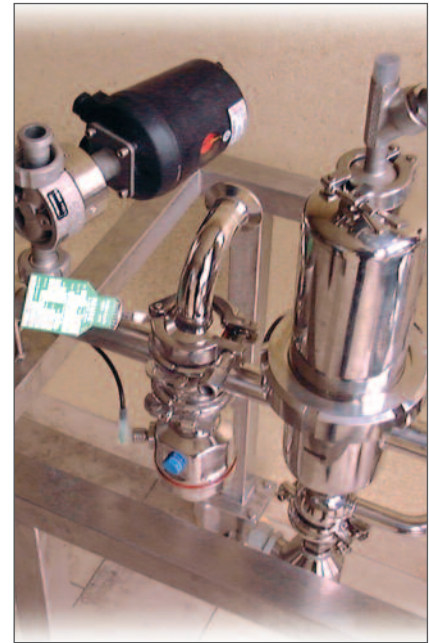
TC(R)-KUB® in test facility
