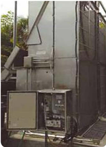
Waste water treatment
