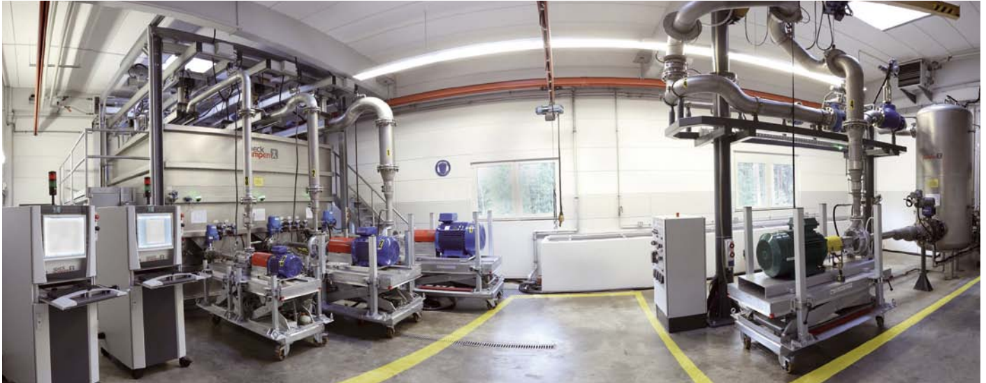
Computer-controlled and fully automated test stands on the premises of Speck in Roth. Measuring of hydraulics, power requirements, axial thrust, vibrations and NPSH values. Heads of up to 400 m and flow rates of up to 750 m 3 /h are possible.
